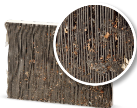
Without A/C maintenance
